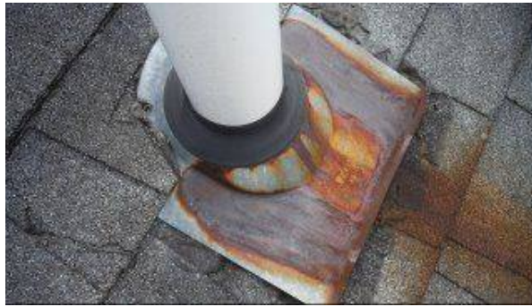
Photo 14-2 Rusting plumbing vent roof jack
