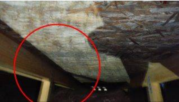
Photo 41-1 Microbial staining from unconnected vent stack
