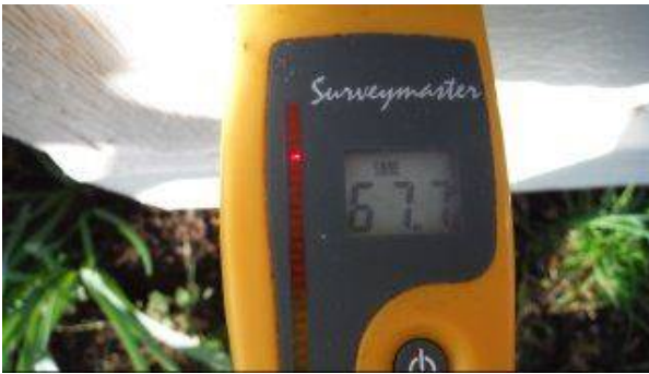
Photo 7-1 Excessive moisture reading at bay window siding.
