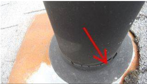
Photo 14-1 Bad neoprene seal
