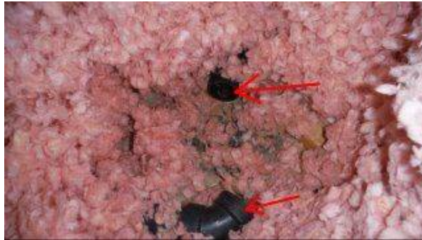
Photo 41-2 Disconnected vent stack
