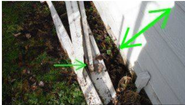
Photo 10-2 Rotten wood should be removed from area as well as the damaged siding and trim.
