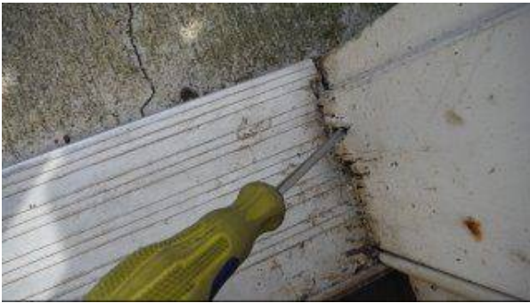
Photo 12-1 Rot at door jambs
