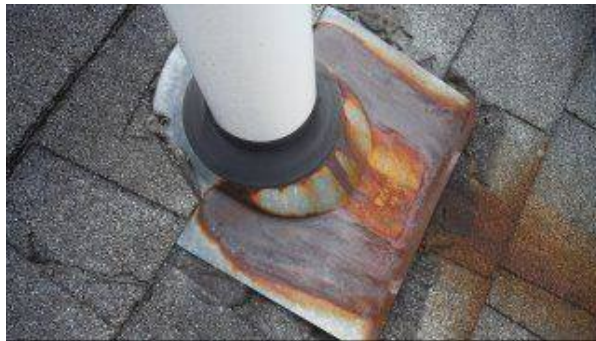
Photo 14-2 Rusting plumbing vent roof jack
