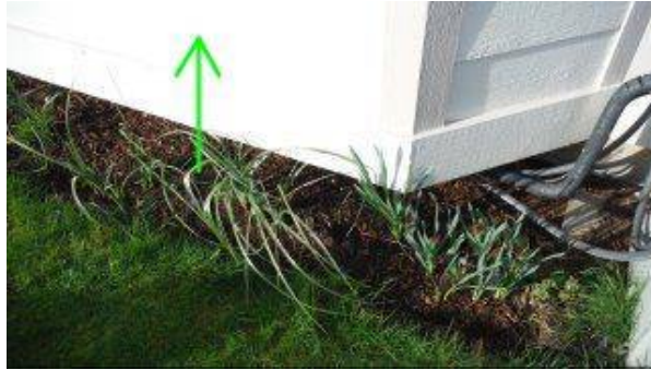
Photo 7-2 Area of damaged siding.
