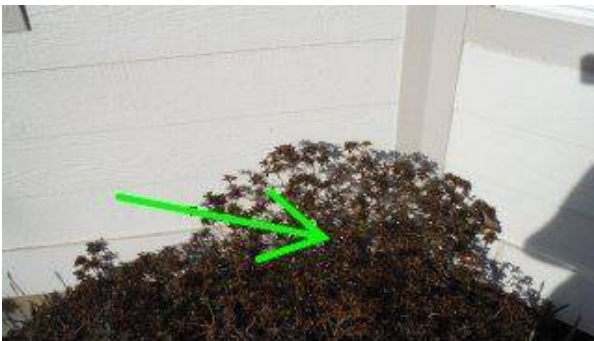
Photo 9-1 Vegetation too close to siding
