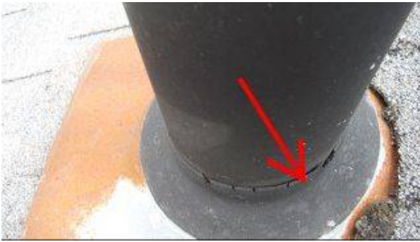
Photo 14-1 Bad neoprene seal
