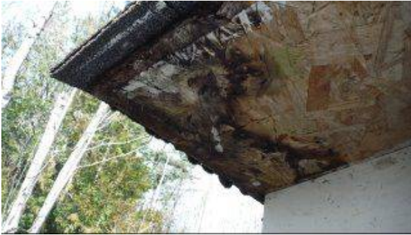
Photo 11-1 Damaged area of roof sheathing and trim.
