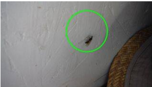
Photo 10-3 Carpenter ants found inside garage
