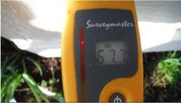
Photo 7-1 Excessive moisture reading at bay window siding.
