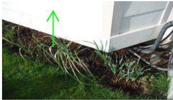
Photo 7-2 Area of damaged siding.
